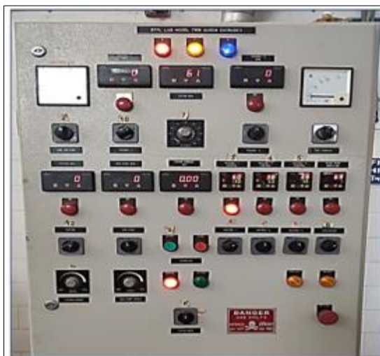
Twin Screw Extruded with the control Panel
